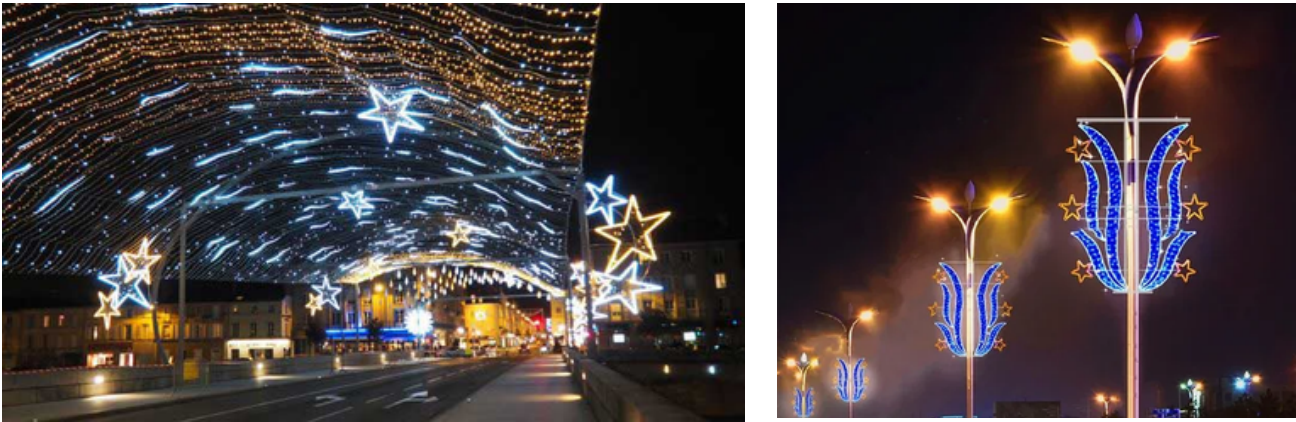
Figure 4.3 Reference Image for Decorative lighting
