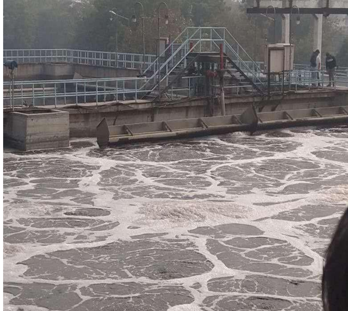
Photograph of STP plant
