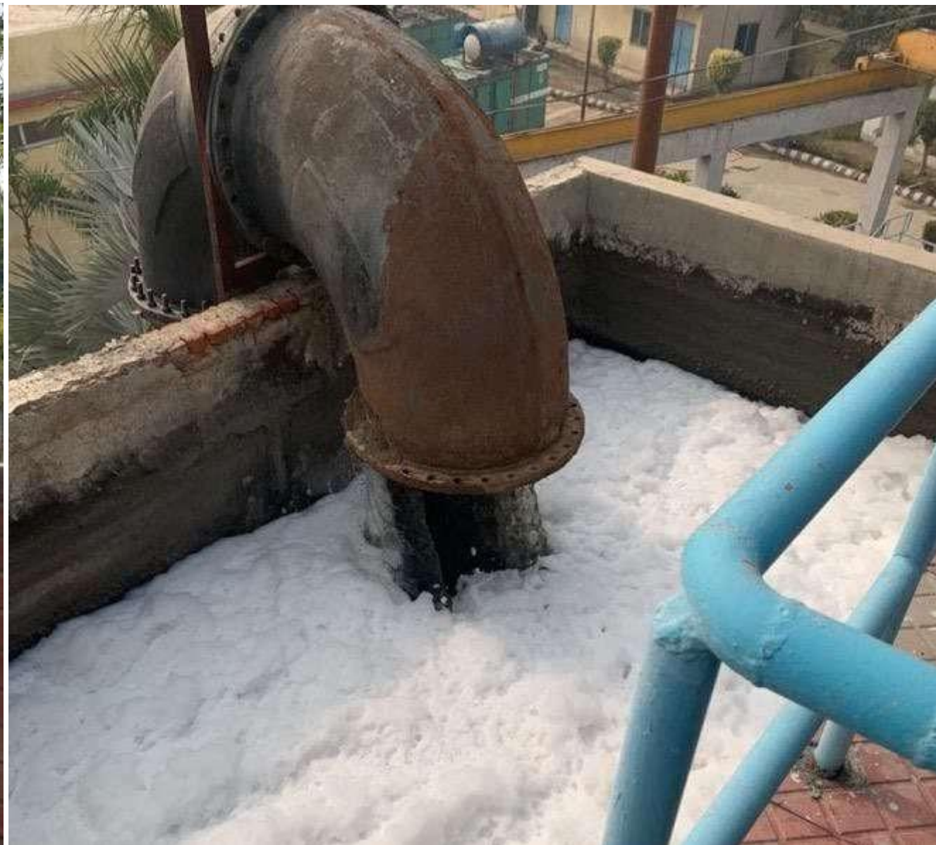
Photograph of inlet sewage
