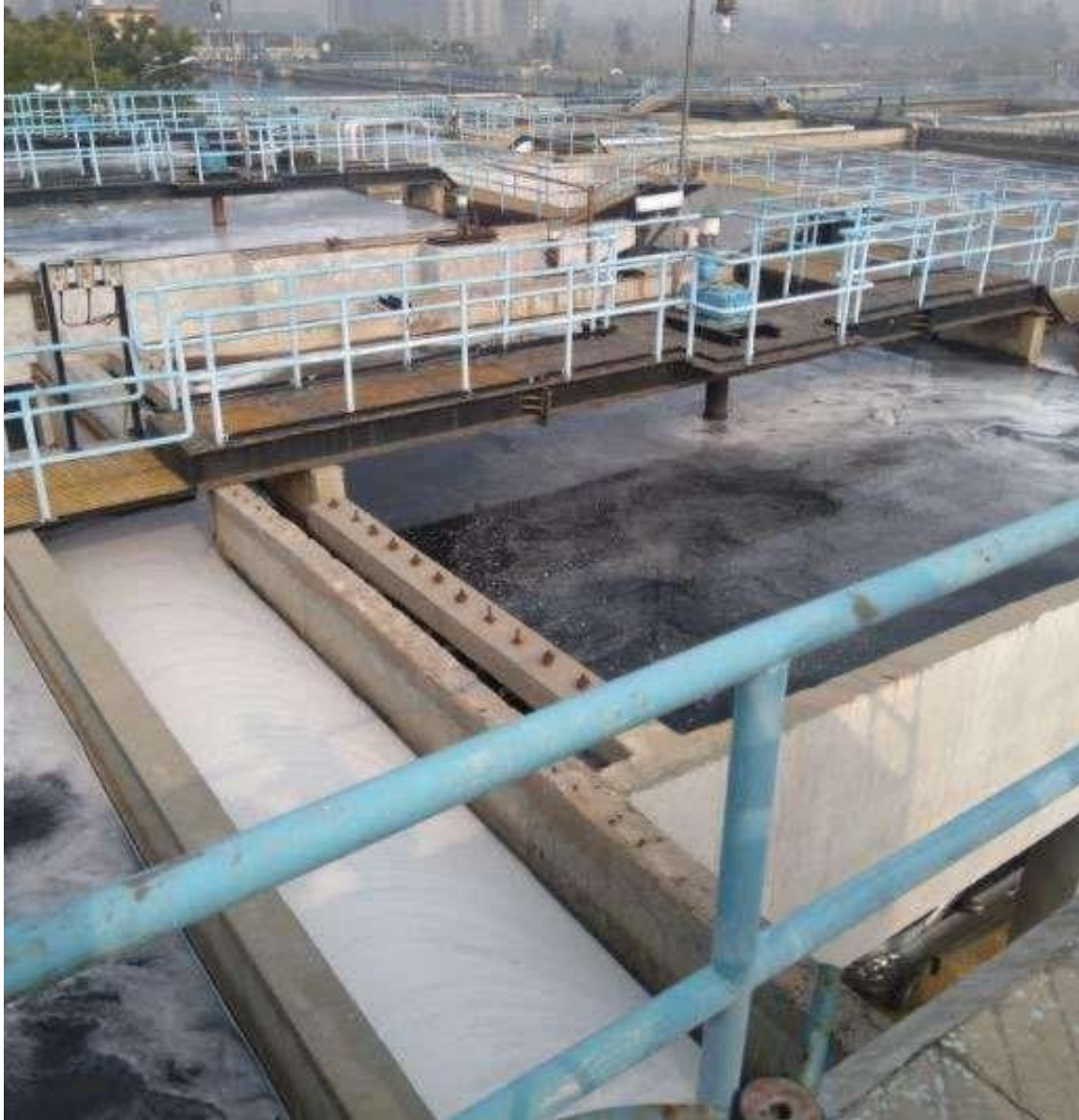
Photograph of STP plant
