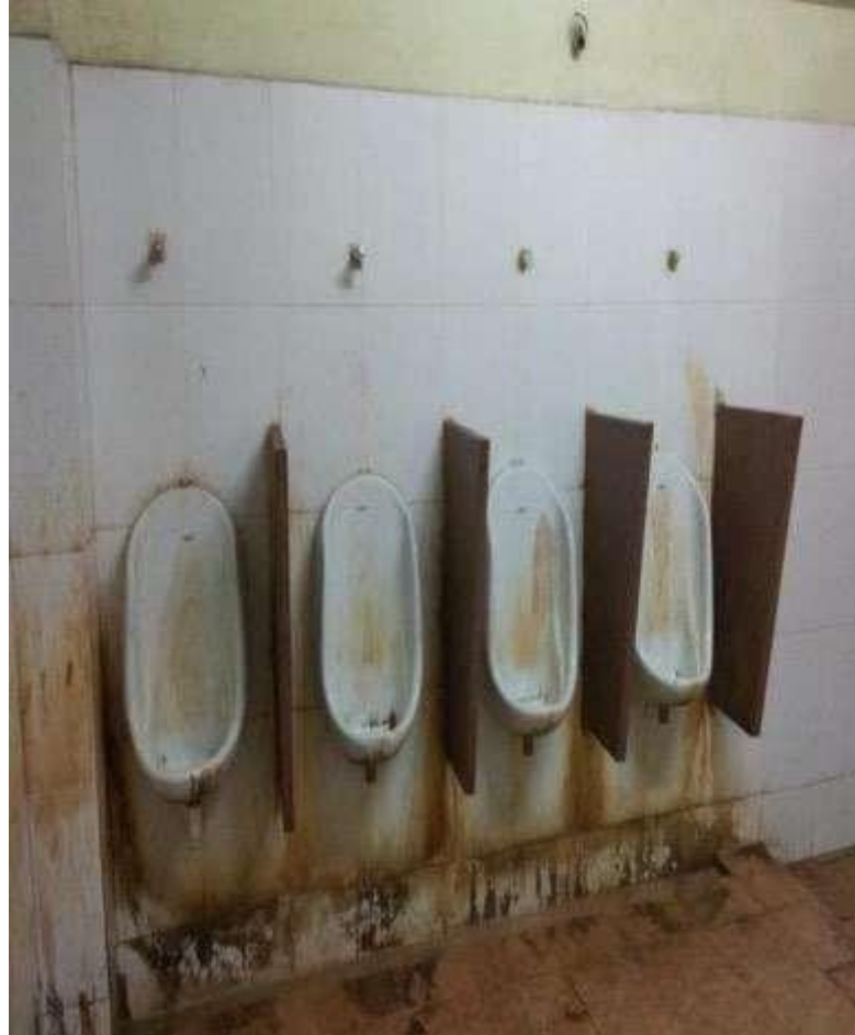
Urinal not clean
