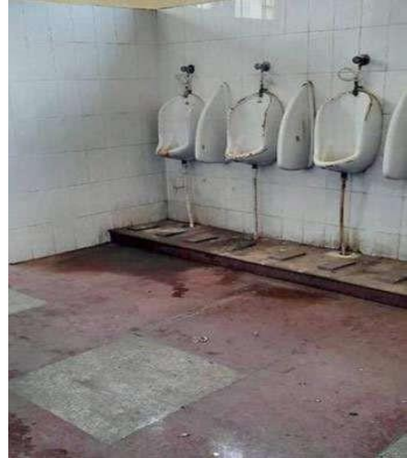
Toilet floor is not clean
